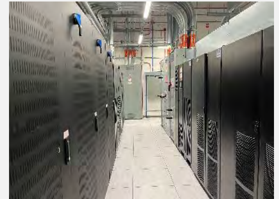
IT Infrastructure at Eisenhower Ave Office
