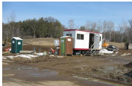
Example of Poorly Maintained Vehicular Route Stabilization
