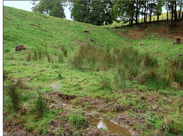
Earthen dam seepage
