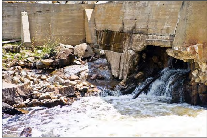
Piping flow through the dam as a result of dam concrete failure
