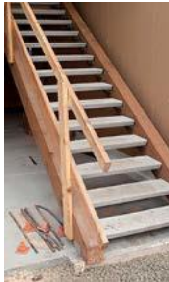
Figure 6. Stairrail System with handrail.
