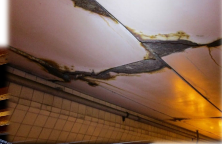
Corroded Steel Sheeting in the Underside of Ceiling Panel
