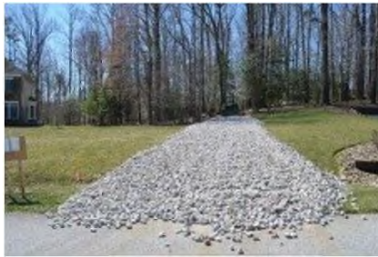
Improperly Maintained Stone Construction Entrance- Stones Dislodged Spilling into Adjoining Roadway
