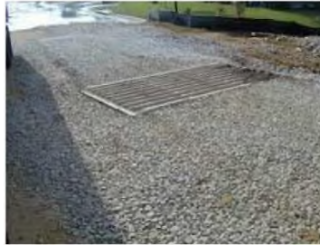
Stone Construction Entrance with Washrack
