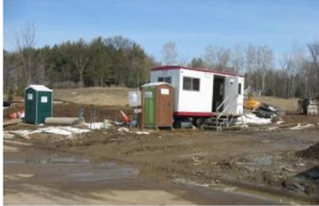
Example of Poorly Maintained Vehicular Route Stabilization
