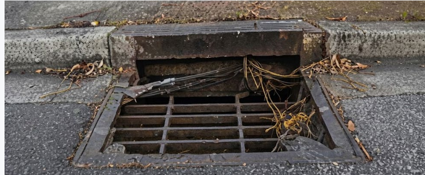
Storm Drains Damage
