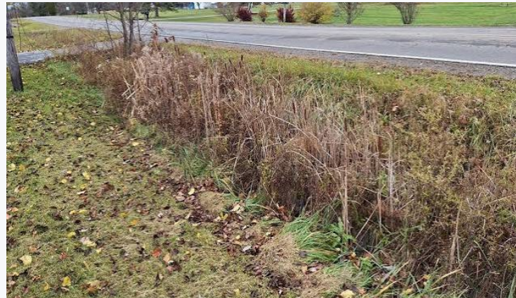
Obstruction of cross-section
