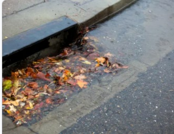
Storm Drains Obstruction
