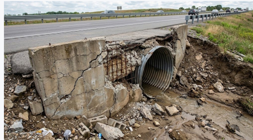
End wall in poor condition
