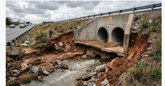
Erosion at outfall
