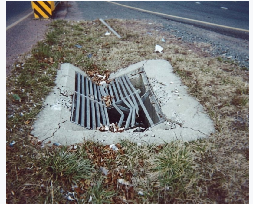
Drop Inlet Damage
