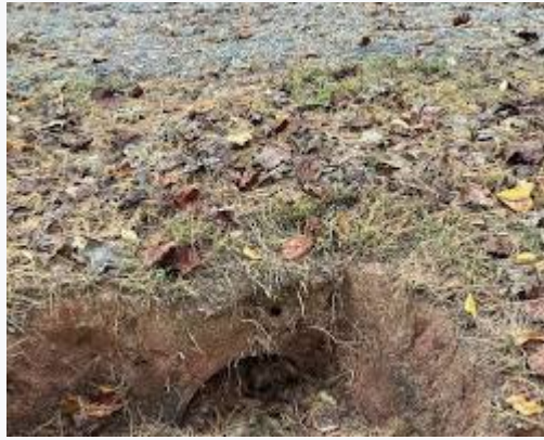
Obstruction of pipe opening
