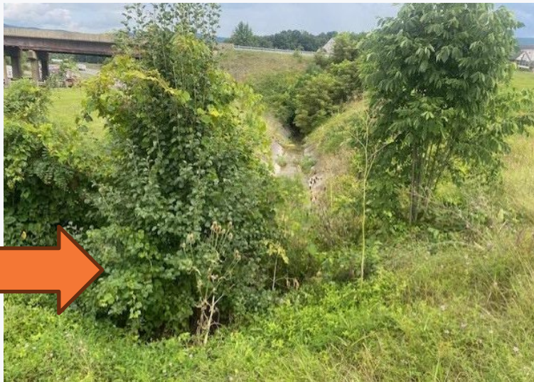
Obstruction of cross-section
