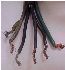
Disconnected wire set
