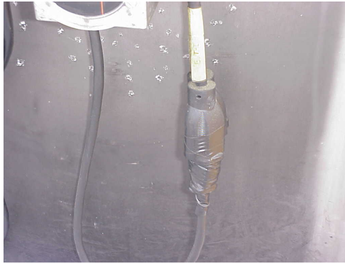
Sealed and taped electrical plug.
