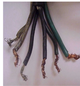
All 3 sets disconnected
