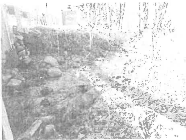
Stream Bank Erosion (No Protection)
