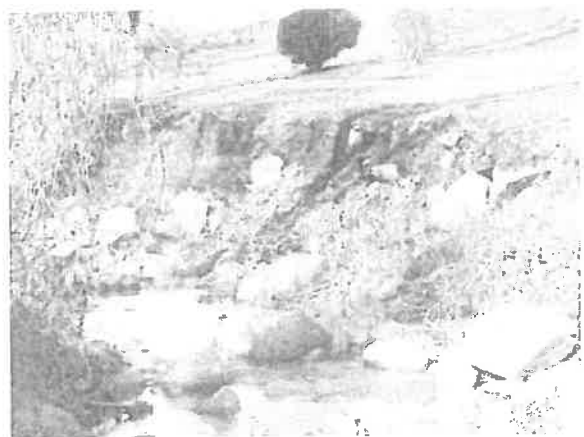
Stream Bank Erosion (No Protection)
