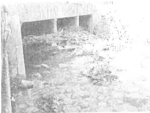
Bridge Abutment Blockage
