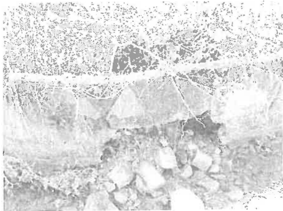
Retaining Wall Failure
